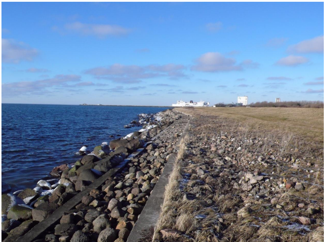
Figure 7.18 Heavily protected dike SE of Rødbyhavn. The revetment is a combined concrete cell and rubble mound structure
