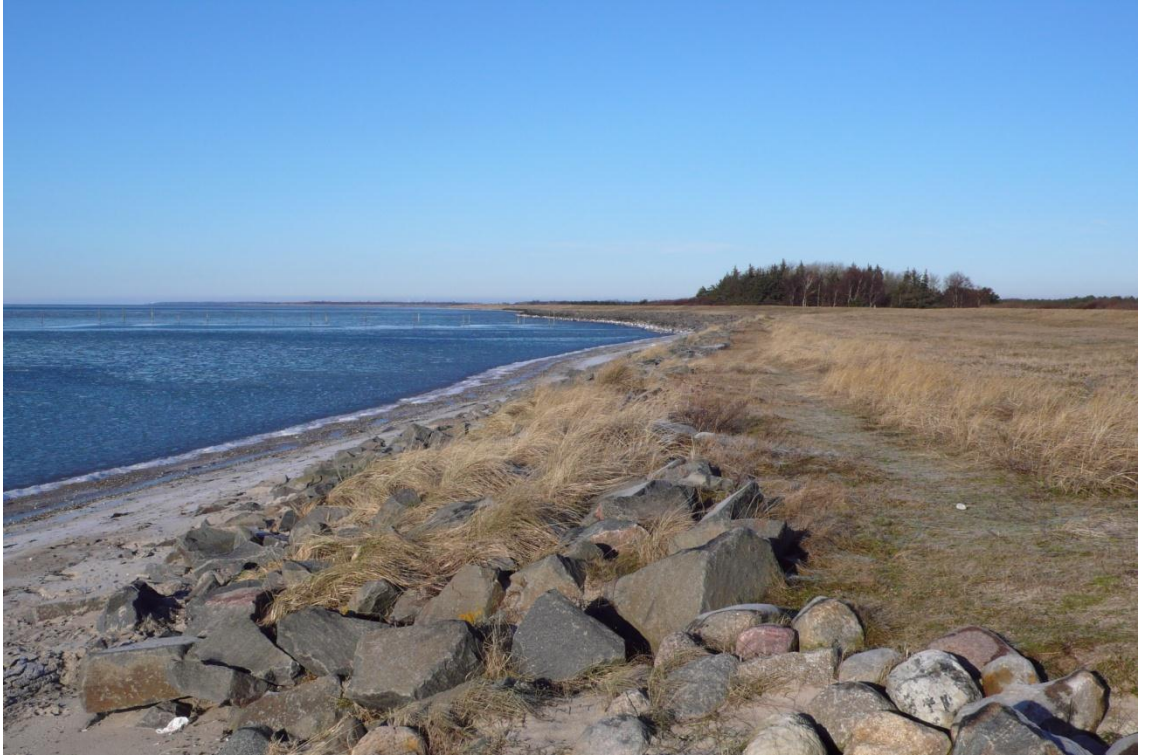
Figure 1.4 Protected section between Skarholm and Bredfjed summerhouse village, photo taken from the west end of the village
